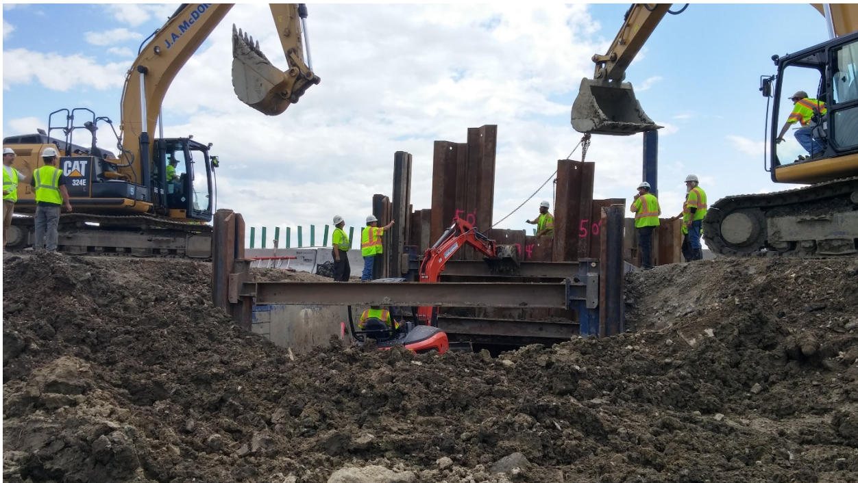
View of excavation of for the new culvert installation just north of the whales tails in So Burlington.
